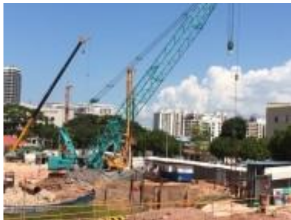
Piling Works for National Centre for Infectious Diseases at Jalan Tan Tock Seng, Singapore
